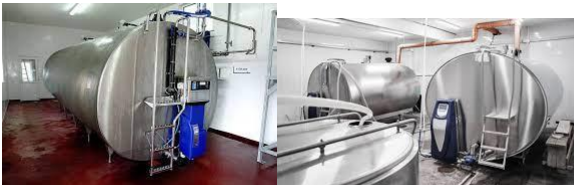
Bulk milk tank in dairy, cannot be removed without knocking wall or removing roof.
